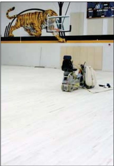
The CHS gym floor is being replaced after a water leak caused it to buckle making it unsafe for play. Basketball games are being played at the middle school gym until the floor is completed January 21.
